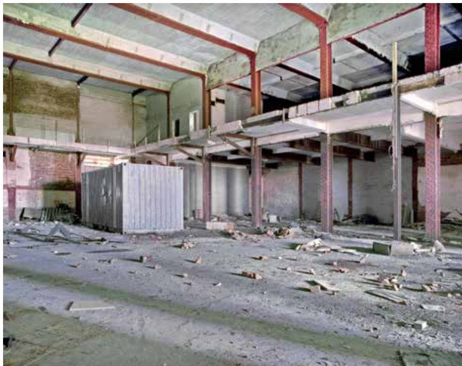
The site of the operations room in June 2004. Most of the internal walls in the two-storey section were removed in 1990 when the building was being converted into a furniture warehouse. This view is looking towards the site of the dais. The upper level gallery is seen. Photo Nick Catford
